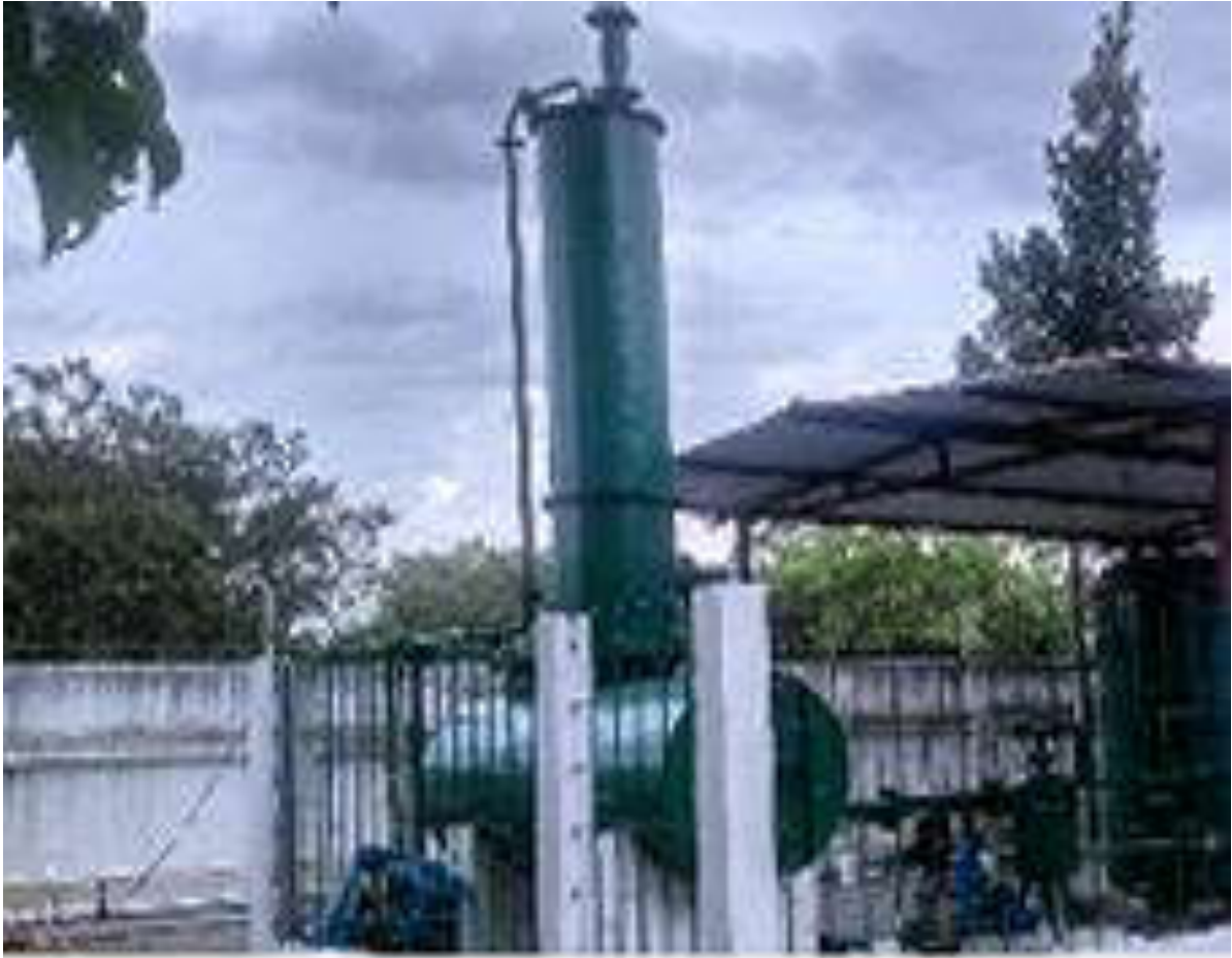
Fig. 3 Water treatment plant of Nazir Ajmal Memorial College of Education
